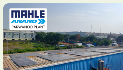
690kW | Himachal Pradesh
