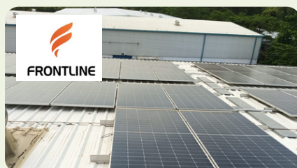
350 kW | Andhra Pradesh
